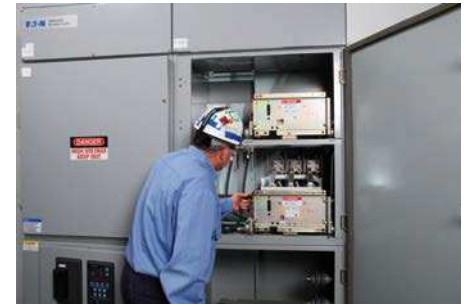
Arcflash Reduction Maintenance System (ARMS)
