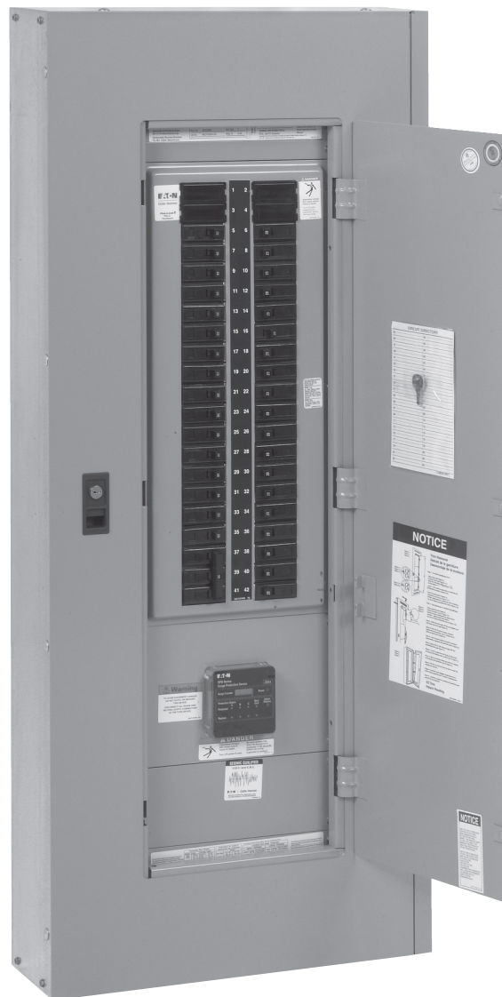
SPD Series Unit Integrated Within an Eaton Panelboard
