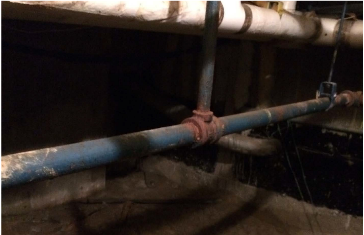
Picture 15. Lead-based and TSCA-regulated PCB blue pipe paint in the Basement, Crawlspace (CAT423-BASE-PC-20).
