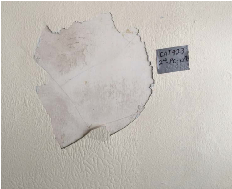
Picture 4. Lead and PCB-containing beige over blue wall paint in the Second Floor, Watershed Division Engineer's Office (CAT423-2ND-PC-04).
