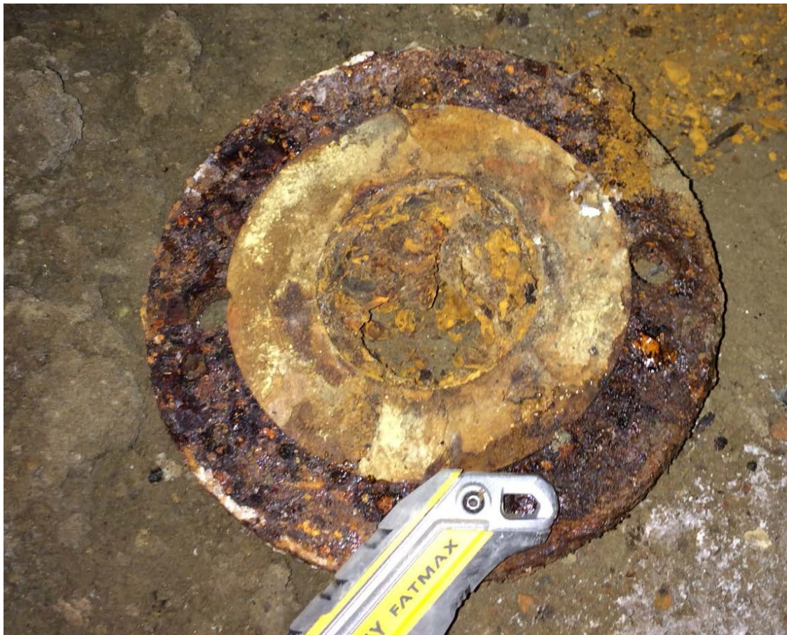
Picture 24. Asbestos-containing brown 4" gasket in the Basement, Crawlspace (CAT423-BASE-ASB-94,95).
