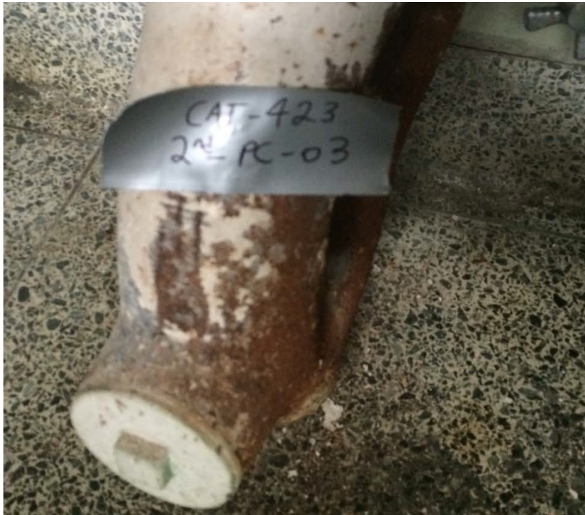
Picture 3. Lead and PCB-containing white sink drain paint in the Second Floor, Men's Bathroom (CAT423-2ND-PC-03).
