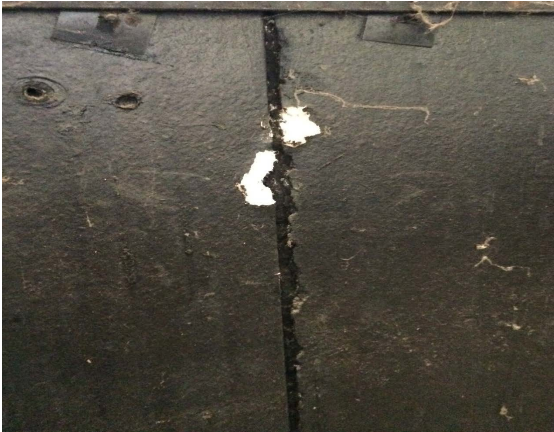
Picture 21. Asbestos-containing black radiator shielding in the Second Floor, Stairwell (CAT423-2ND-ASB-28,29).
