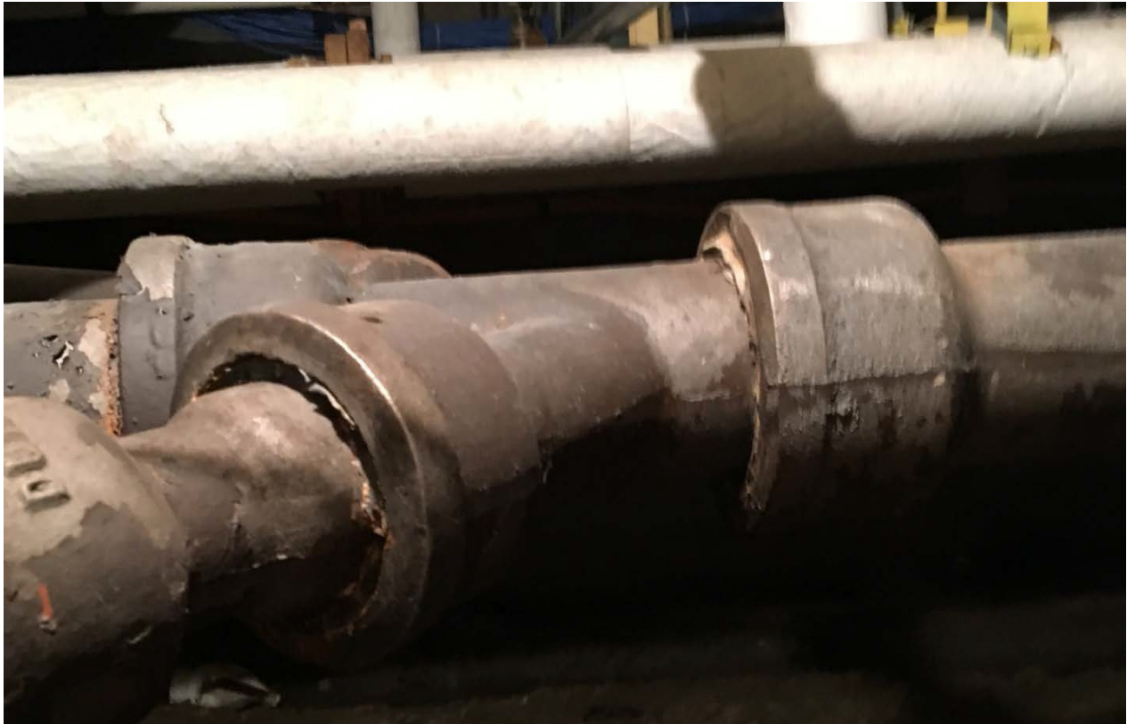
Picture 14. Lead-based and TSCA-regulated PCB brown drain pipe paint in the Basement, Crawlspace (CAT423-BASE-PC-19).
