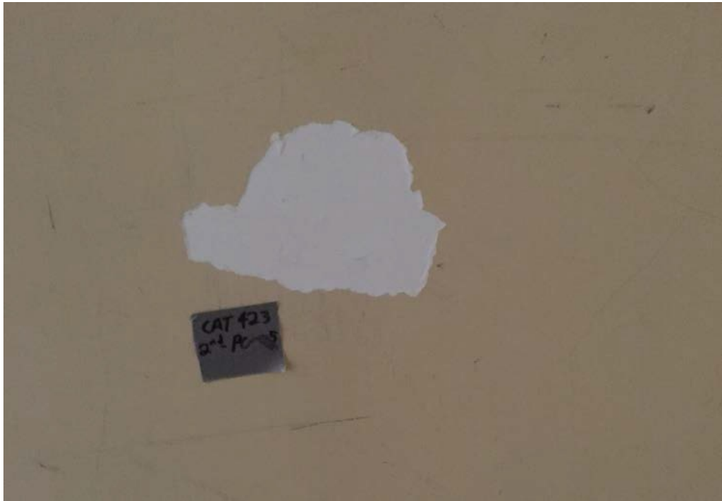
Picture 5. Lead and PCB-containing yellow wall paint in the Second Floor, Watershed Engineer's Office closet (CAT423-2ND-PC-05).
