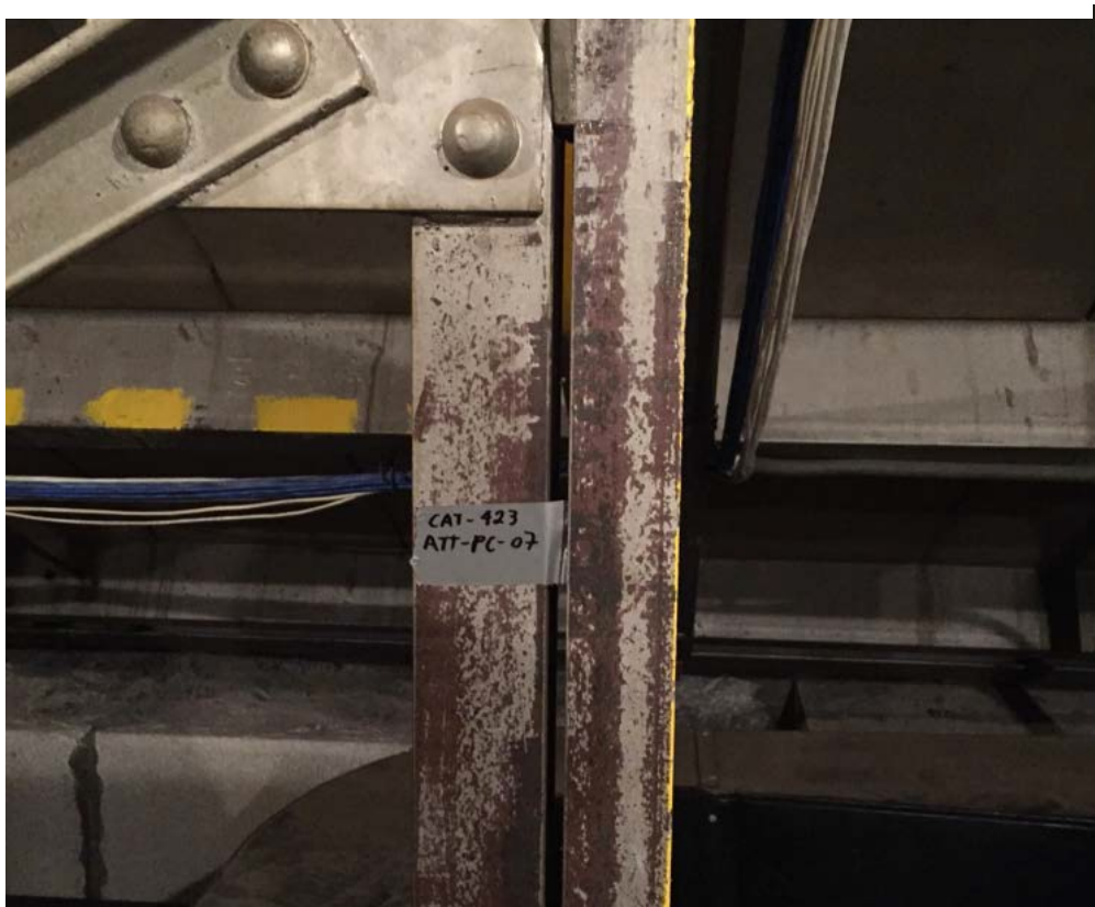
Picture 6. Lead-based and PCB-containing silver framework paint in the Attic (CAT423-ATT-PC-07).
