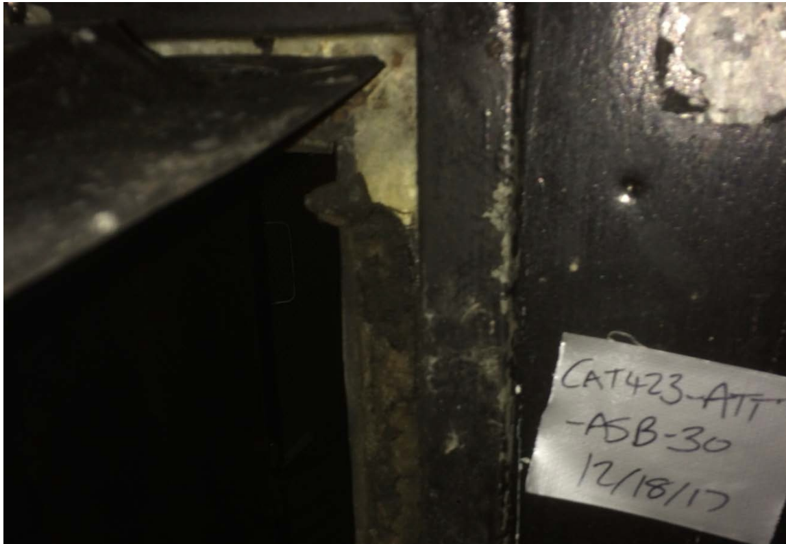
Picture 25. Gasket in Attic HVAC unit containing trace asbestos (CAT423-ATT-ASB-30).
