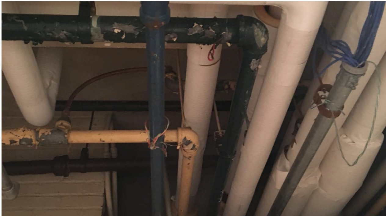
Picture 16. Lead-based and TSCA-regulated PCB green and yellow paints on pipes in the Basement, Storage Room (CAT423-BASE-PC-21,22).
