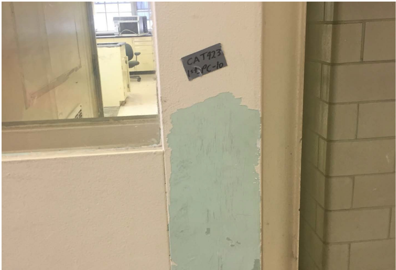
Picture 7. Lead and PCB-containing beige over green door paint in the First Floor, Office (CAT423-1ST-PC-10).
