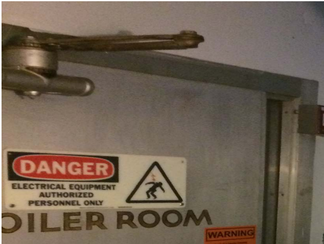
Picture 19. Door Closer with PCB-containing oil on Basement, Boiler Room Door (CAT423-1ST-PCB-11)
