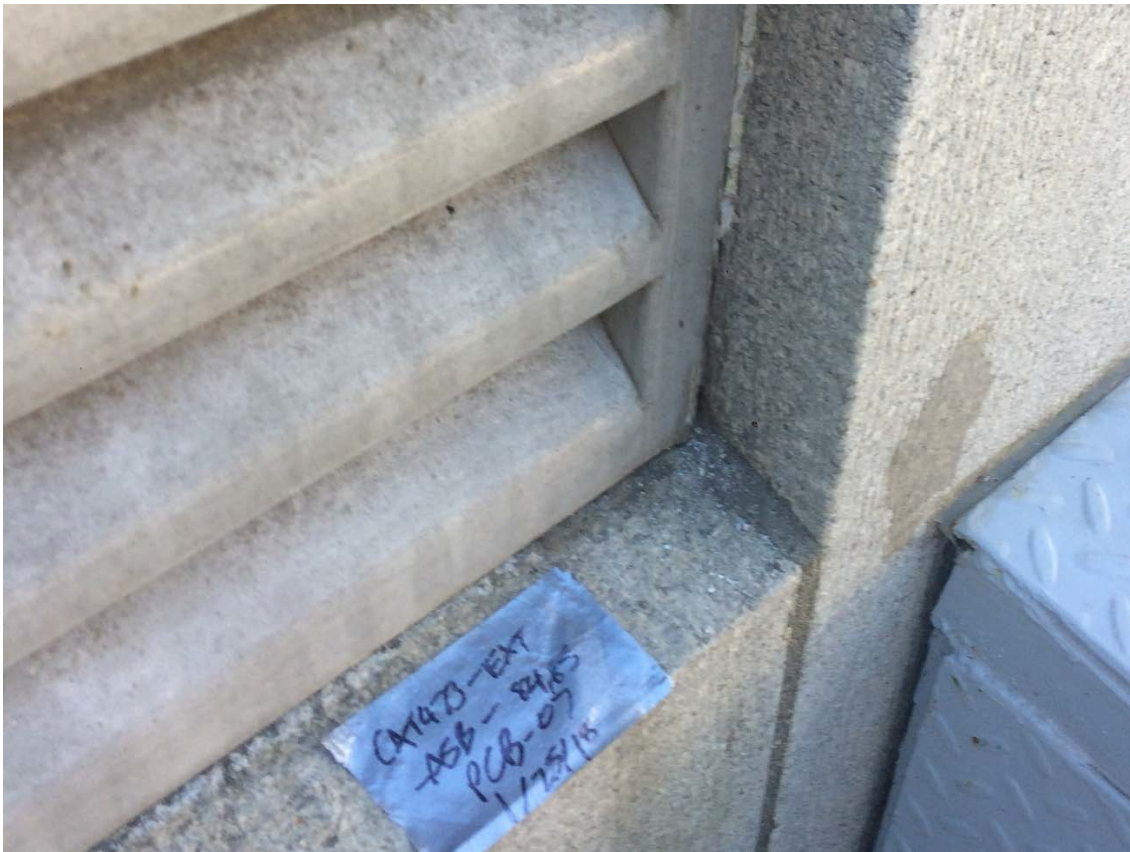
Picture 23. Asbestos-containing white caulk around Exterior, South Wall vent (CAT423-EXT-ASB-84,85).
