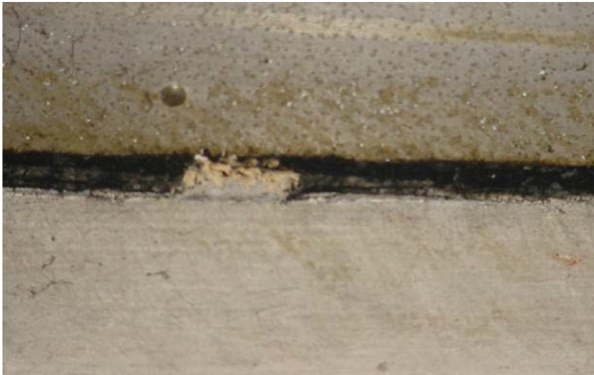
Picture 18. PCB-containing caulk around the Basement, Boiler Room door (CAT423-BASE-PCB-02).
