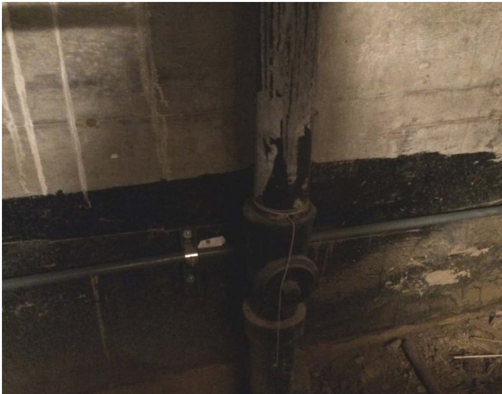
Picture 13. Lead-based and TSCA-regulated PCB black drain pipe paint in the Basement, Crawlspace (CAT423-BASE-PC-18).
