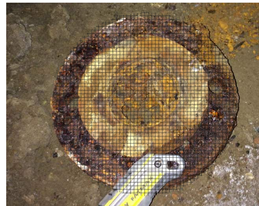
ASBESTOS-CONTAINING BROWN 4" GASKET IN THE BASEMENT, CRAWLSPACE (CAT423-BASE-ASB-94,95).
