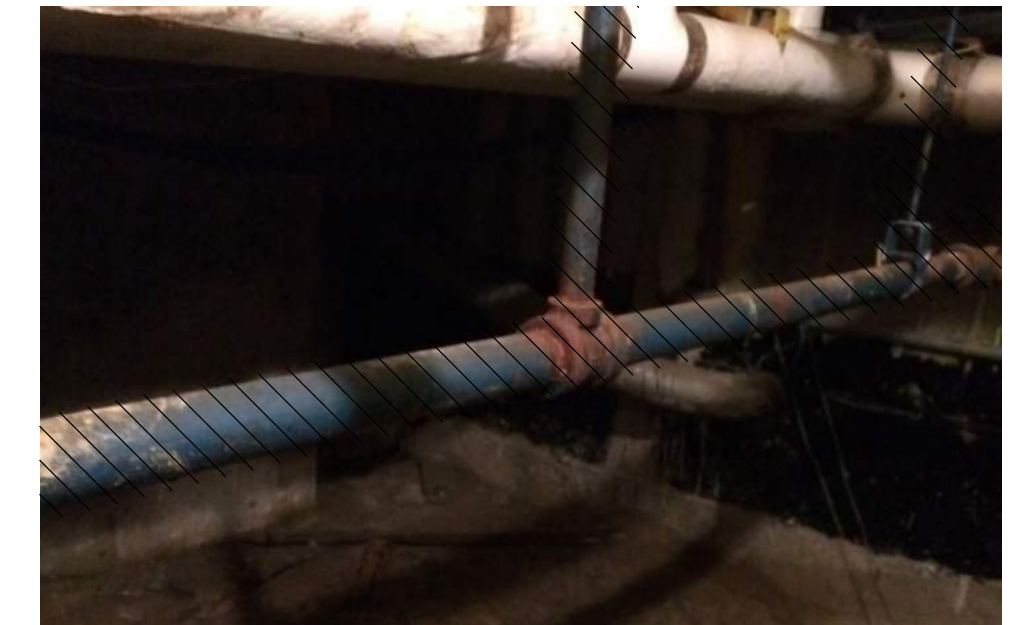
LEAD-BASED AND TSCA-REGULATED PCB BLUE PIPE PAINT IN THE BASEMENT, CRAWLSPACE (CAT423-BASE-PC-20)
