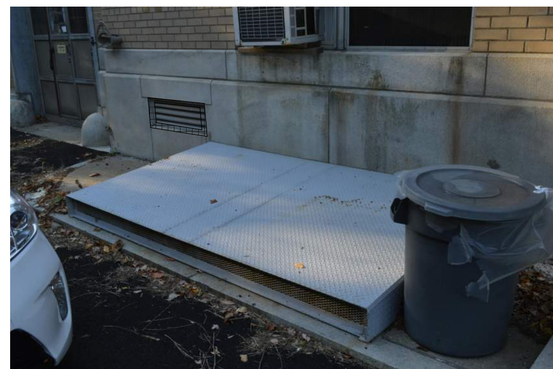
ASBESTOS CONTAINING WHITE CAULK AROUND EXTERIOR VENT, TYP. (CAT423-EXT-ASB-84, 85)
