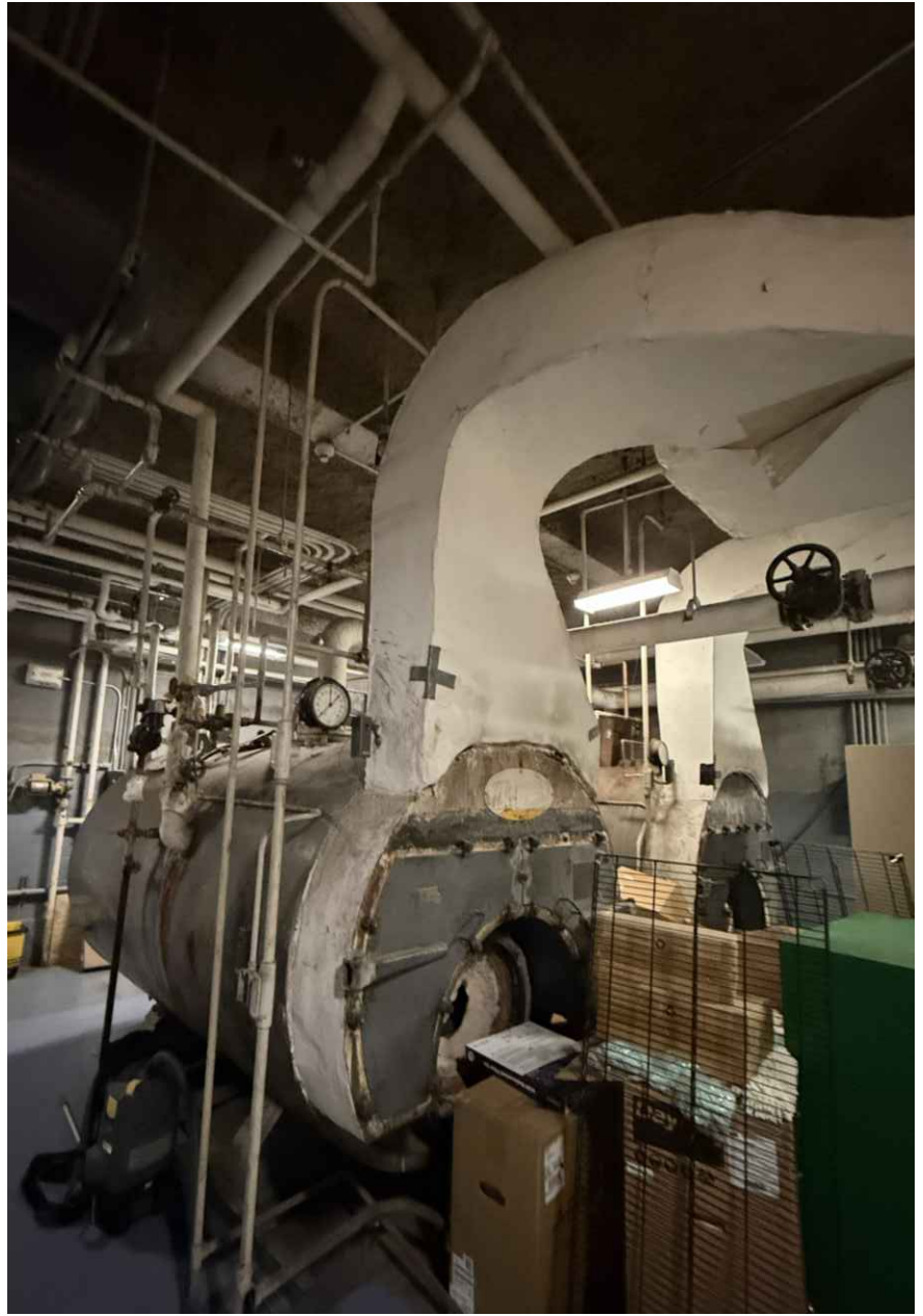
BOILER ROOM PICTURE
