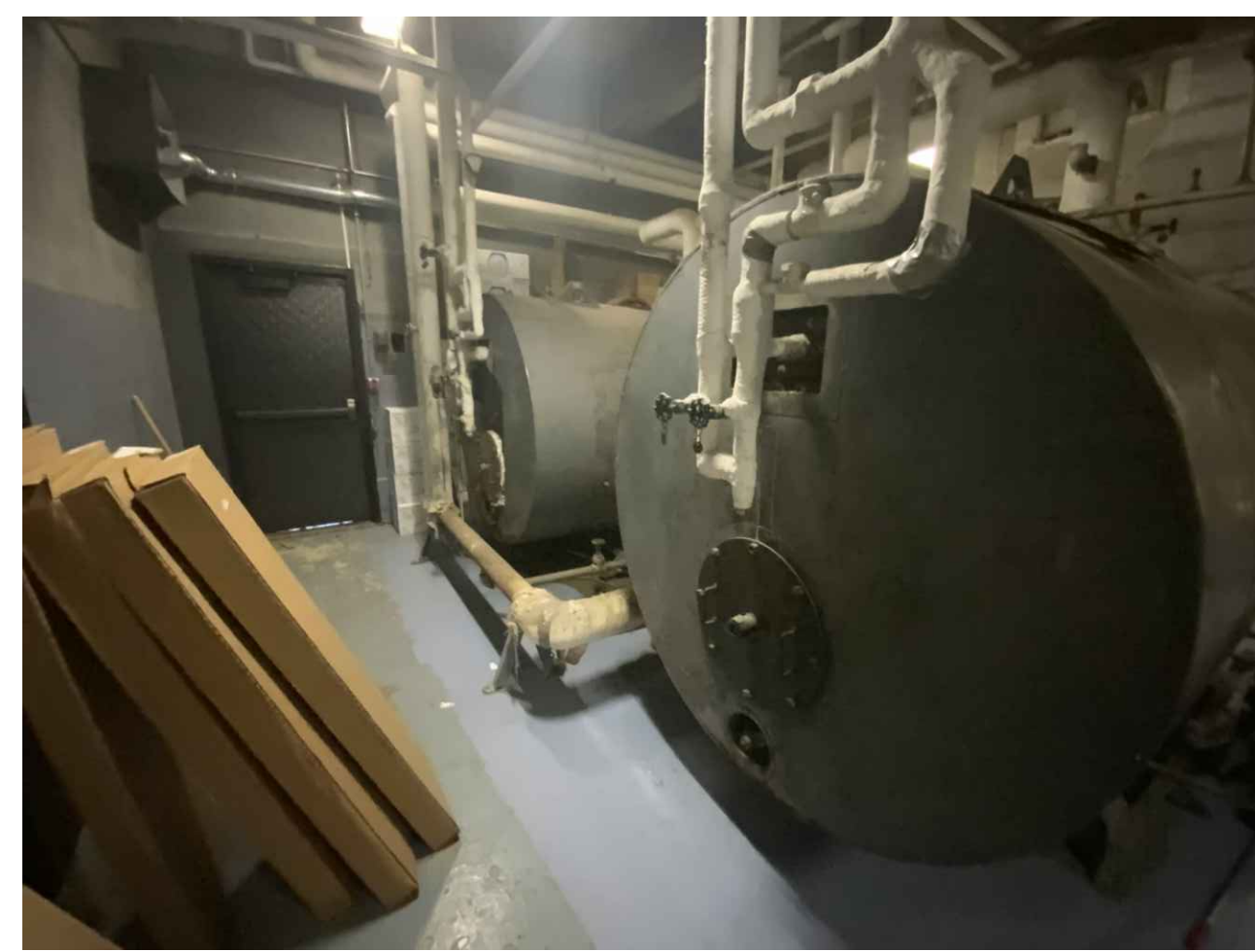
BOILER ROOM PICTURE
