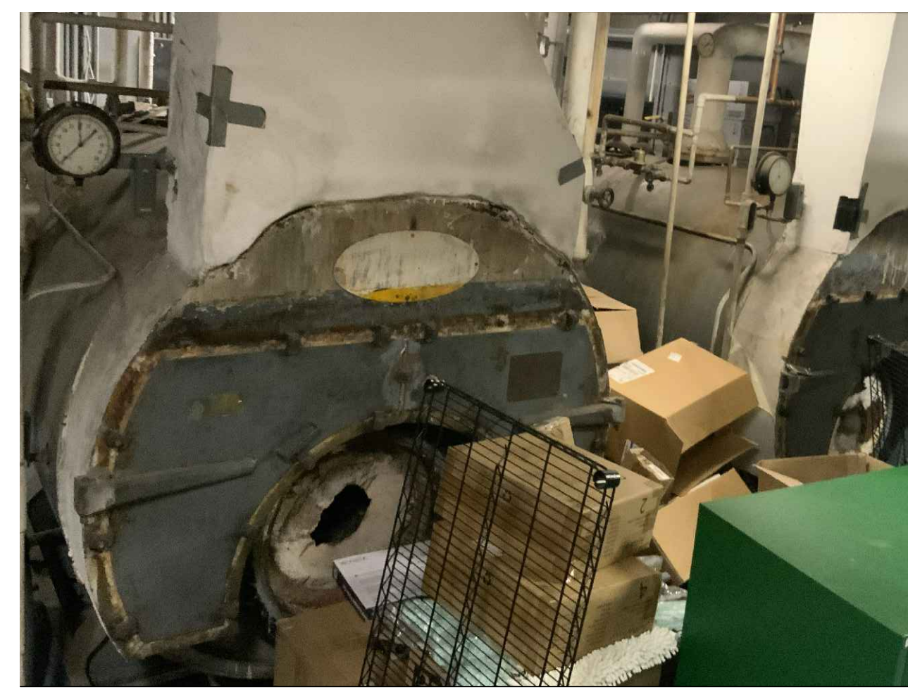
BOILER ROOM PICTURE
