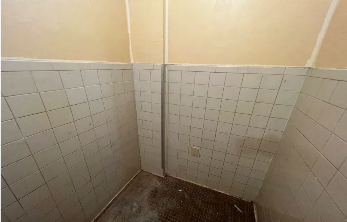
ABOVE: ACM JOINT COMPOUND & CONTAMINATED SHEETROCK (TYPICAL)
