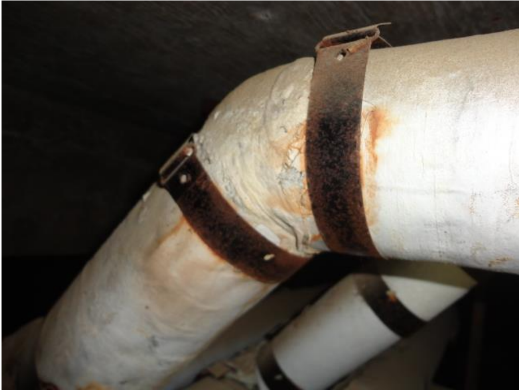
Sample #7 - Mudded Fittings - 23.5% Chrysotile
