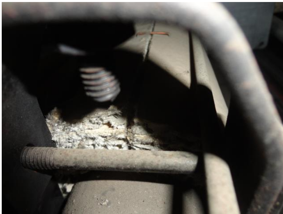
Sample#3 - Brown Paper Insulation - 2.5% Chrysotile
