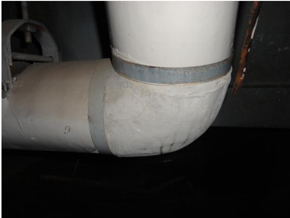
Sample #7 - Mudded Fittings - 66.7% Chrysotile
