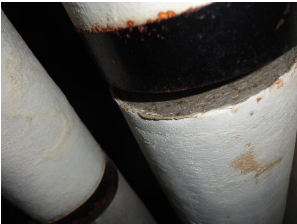
Sample #4 - Layered Pipe Insulation - 2.0% Chrysotile
