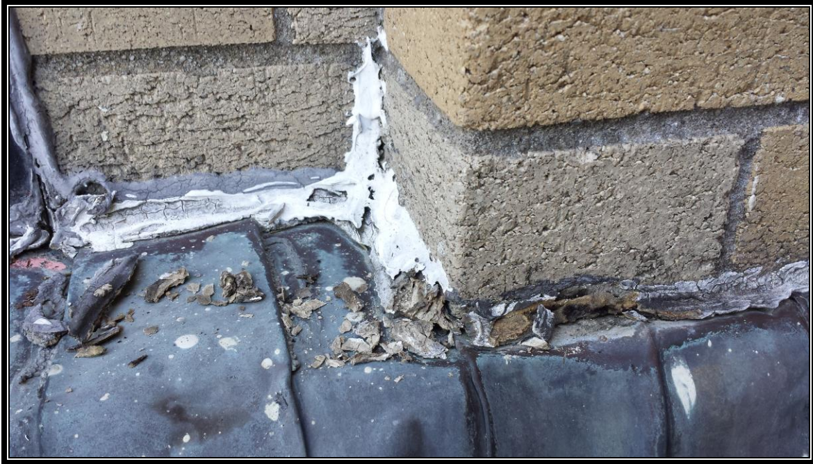
Photograph 1: Caulk Assoc. with Copper Deck/Coping Stone Seam, Cap Flashing Caulk, Old, Cap Flashing Caulk, Dark Grey & Cap Flashing Caulk, White
