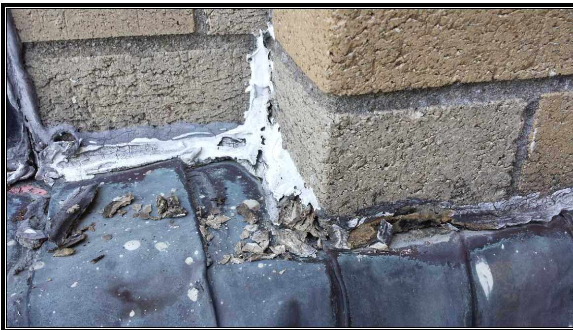
Photograph 1: Caulk Assoc. with Copper Deck/Coping Stone Seam, Cap Flashing Caulk, Old, Cap Flashing Caulk, Dark Grey & Cap Flashing Caulk, White
