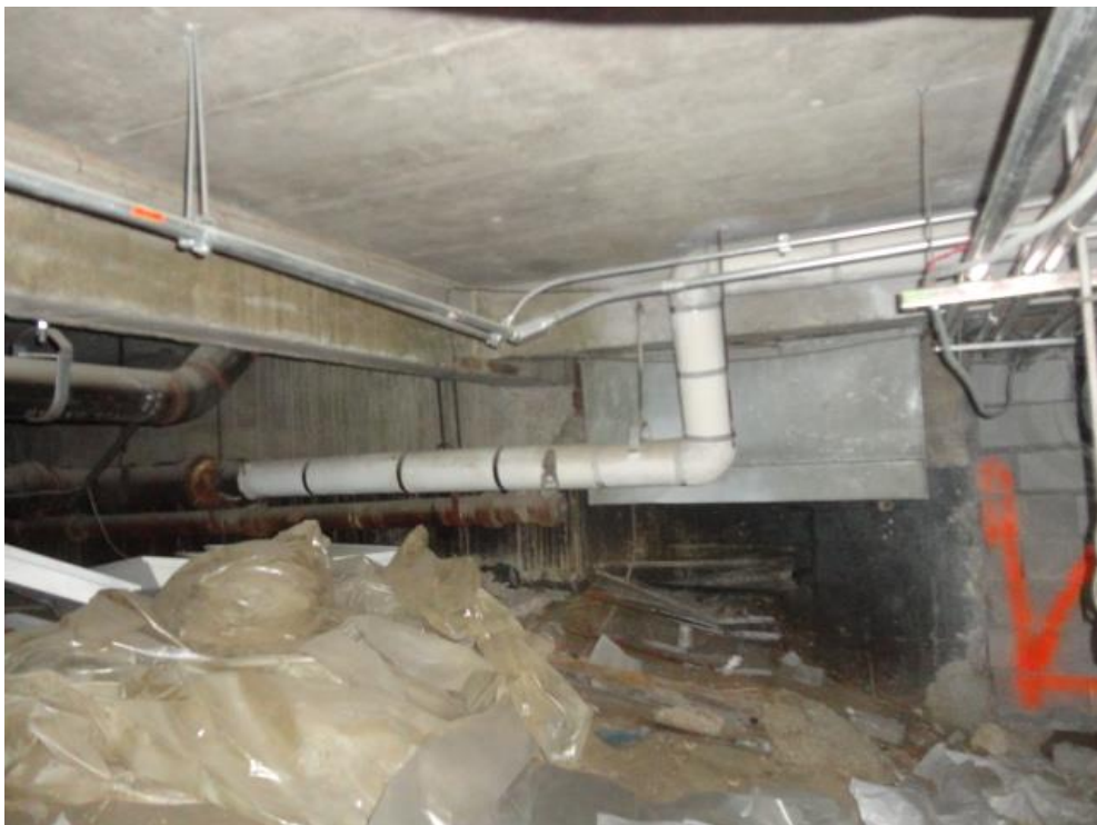
Sample #4 - Layered Pipe Insulation - 1.8% Chrysotile
