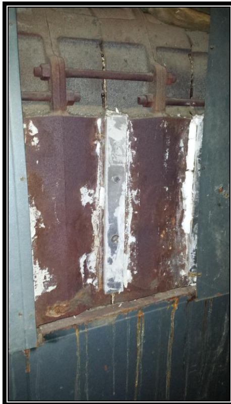
Photograph 2: Cementitious Materials Assoc. with Boiler
