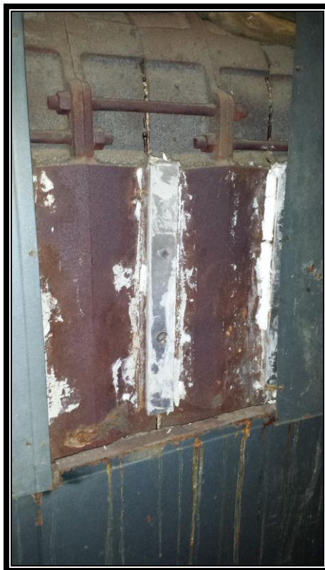
Photograph 2: Cementitious Materials Assoc. with Boiler
